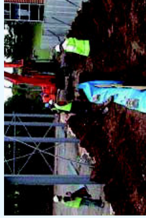
Stage 3: Support the root barrier membrane with shutter ply and backfill the trench.
