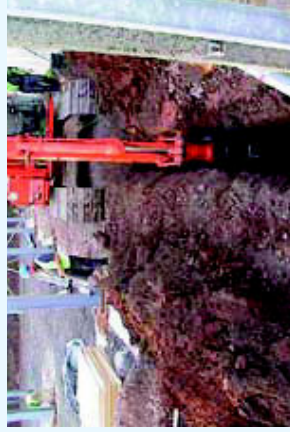
Stage 1: Excavate a trench, making sure that all the knotweed is contained.
